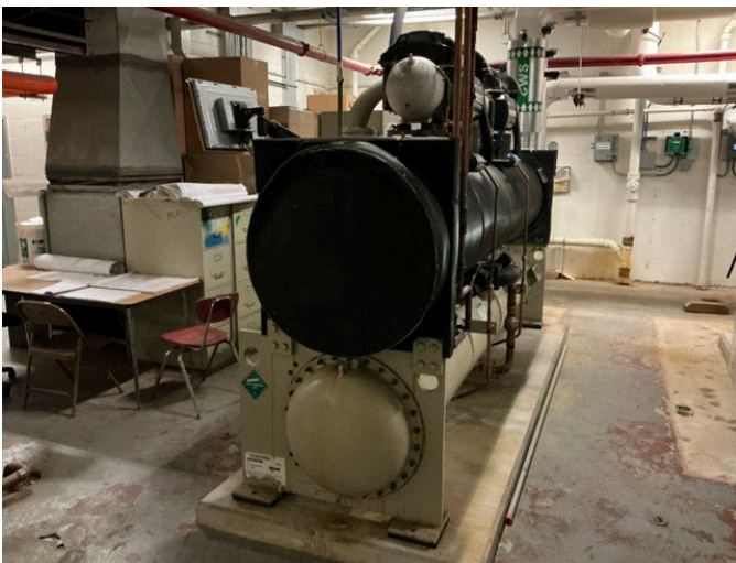
35 - WATER COOLED CHILLER
