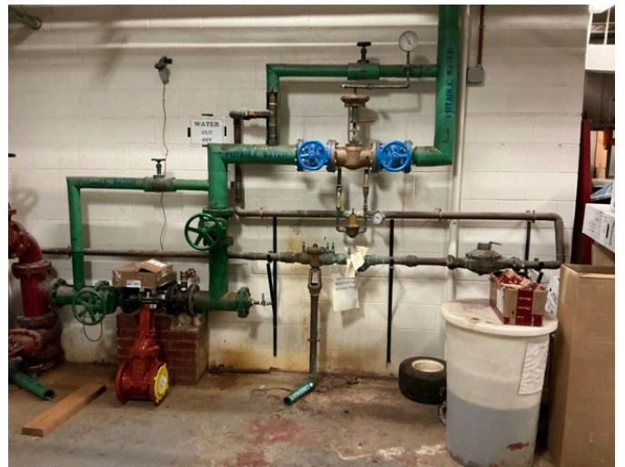
28 - DOMESTIC WATER SERVICE
