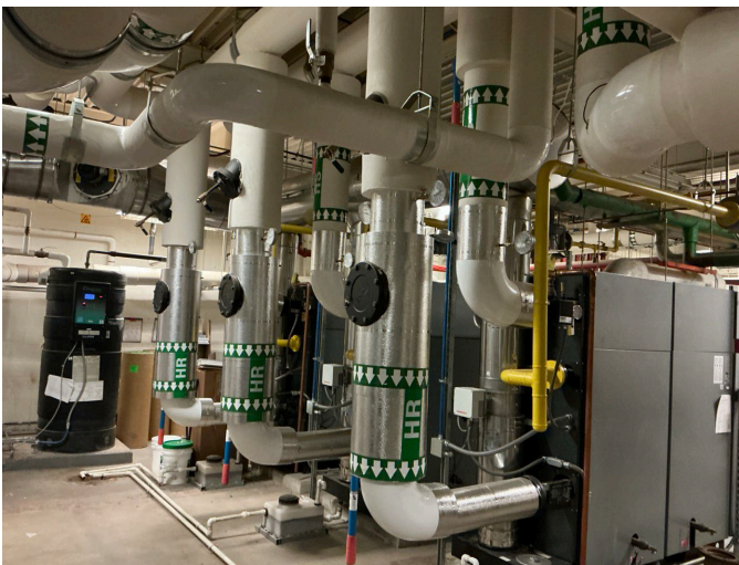
29 - MAIN MECHANICAL ROOM
