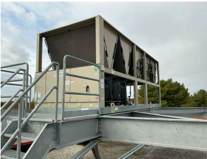
33 - AIR COOLED CHILLER
